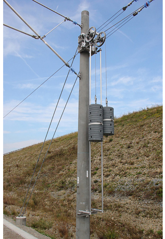
Figure 3: Tension wheel assembly with a mechanical transmission ratio of 1 : 3 and 30 kN operating load, Sicat 8WL5000 on DB's new high-speed line between Leipzig and Erfurt.
