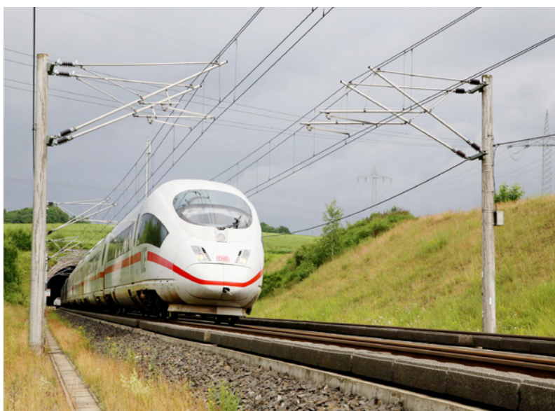
Figure 1: ICE 3 and overhead contact line type Sicat on the high-speed line Cologne – Frankfurt (photo and graphics: SPL Powerlines Germany).
